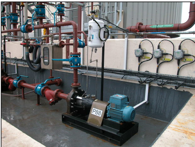
Figure 3 –Amarinth pumping equipment in situ at Nufarm where the production of crop protection products requires equipment to operate in areas designated as ATEX Zone I
