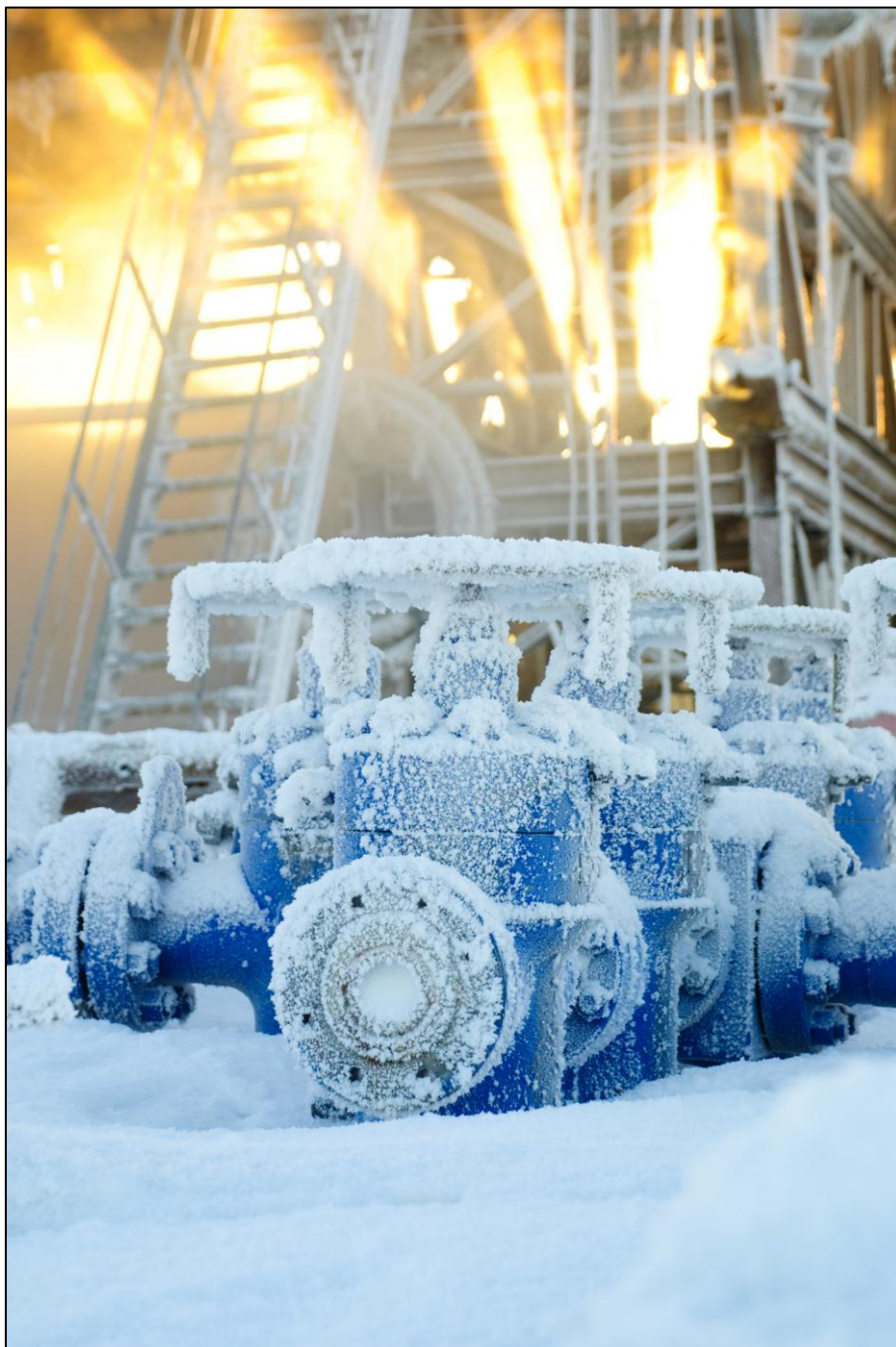
The harsh Sakhalin Island winter requires specialised pumps
