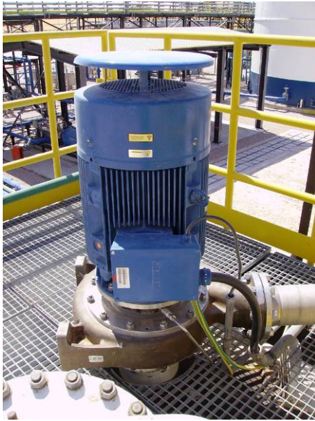
Amarinth pump in-situ
