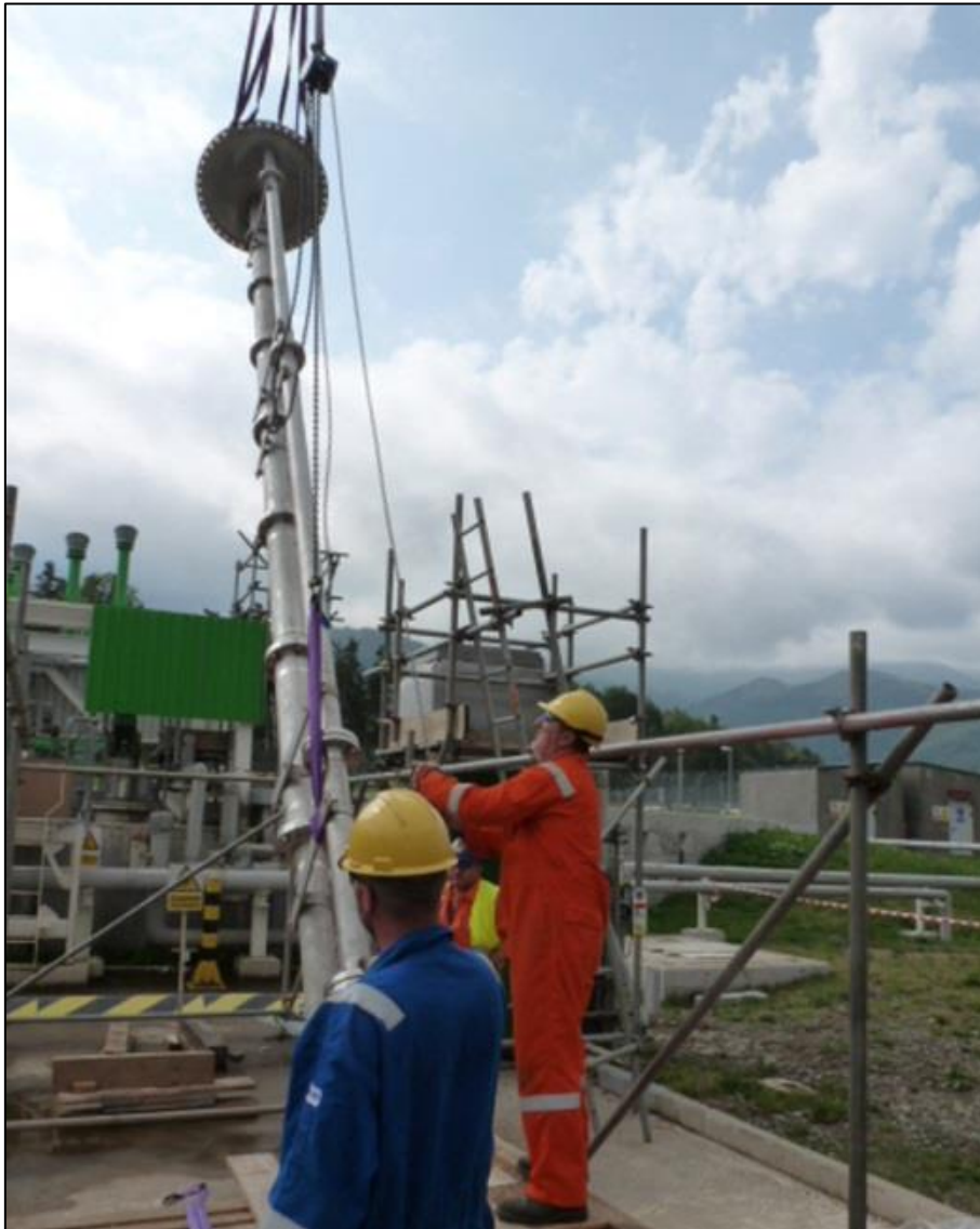
Engineers lifting an Amarith API 610 VS4 pump from a sump station on the Baku-Tbilisi-Ceyhan oil pipeline
