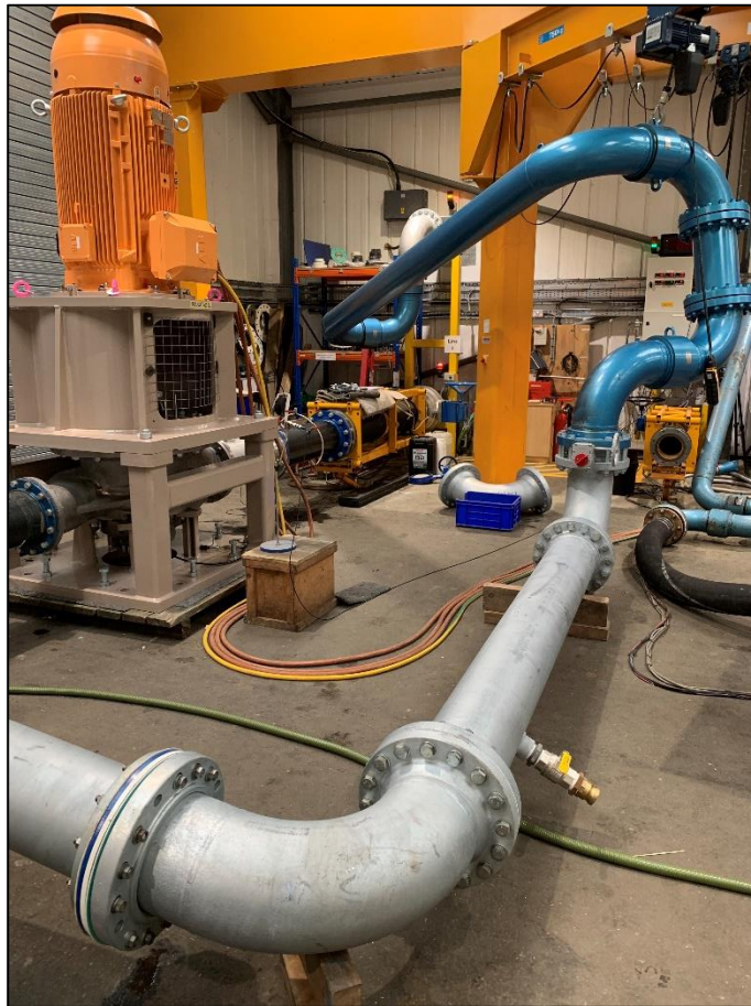
An Amarith in-line vertical pump being tested in the new expanded facilities and destined for a COSCO vessel being built in China
